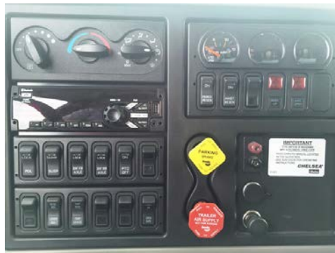
Representative picture of control systems.
